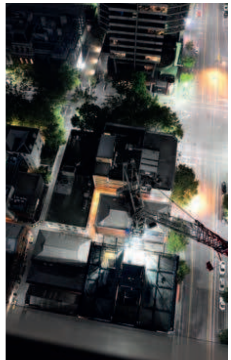
The vertical reinforced steel cages creating a complete floor are lifted into place and locked together during the night by a team of riggers dedicated solely to this task
